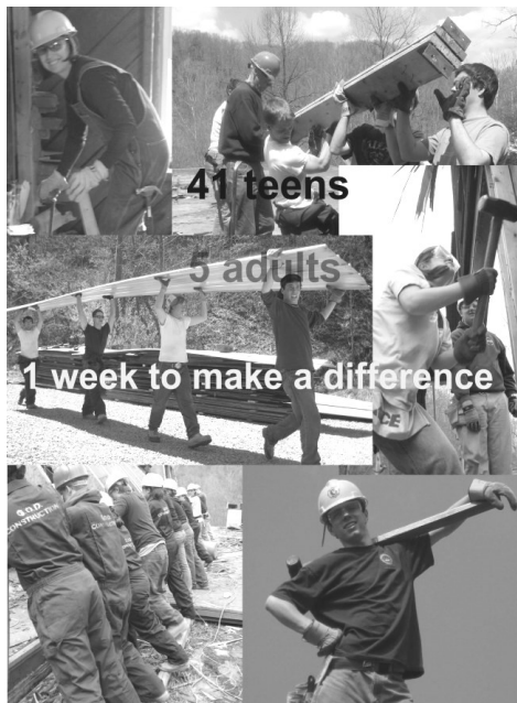
HYG members spend their Spring break building and repairing homes in Kentucky.
